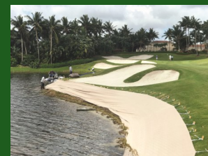
(Golf Course Erosion During)
